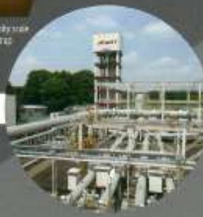
Water flow calibration facility
