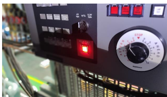
M/E Emergency Trip Test
