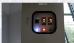
Temperature and humidity monitoring system
