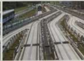
供電軌 Power Rail (3rd Rail)
