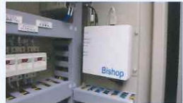
Remote monitoring system
