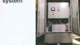
Wastewater monitoring system
