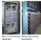
Electronic Interlocking and Relay Interlocking Equipment
