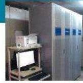
Centralized Electronic Interlocking System
