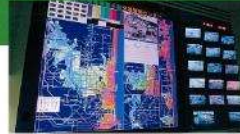
Road Traffic Control System
