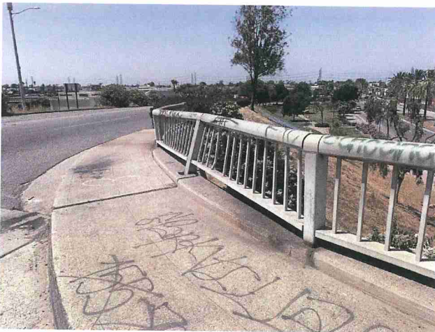
Photo 7 Damage Section of Bridge Rail
