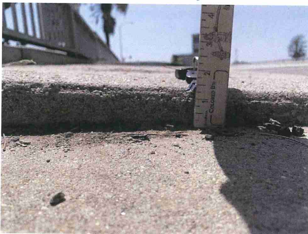
Photo 9 Displacement at SE Approach Sidewalk
