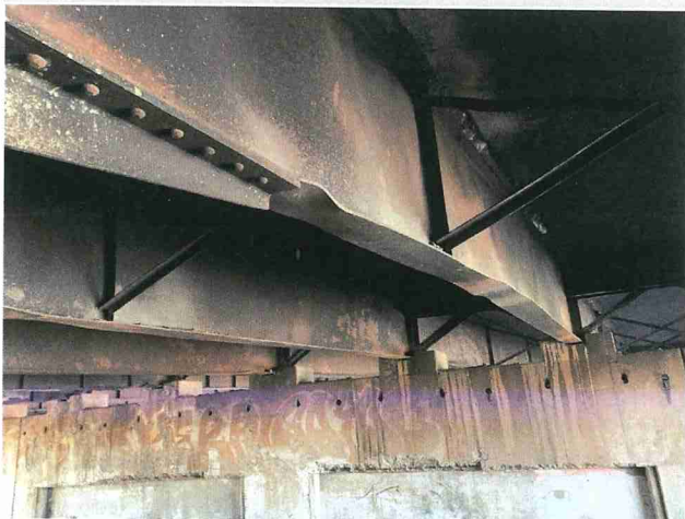
Photo 15 Distorted Lower Flanges and Girder Bracings
