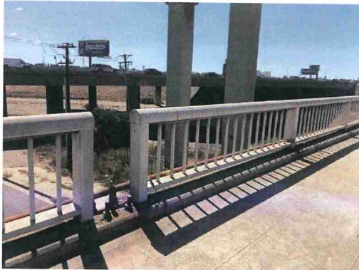
Gap between handrail after utility post was removed _ Need repair (Newfound)
