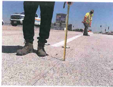
2.5" buckled downward in eastbound roadway portion of span 10
