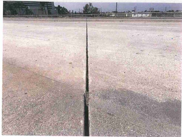
Photo 6 Missing Joint Seal
