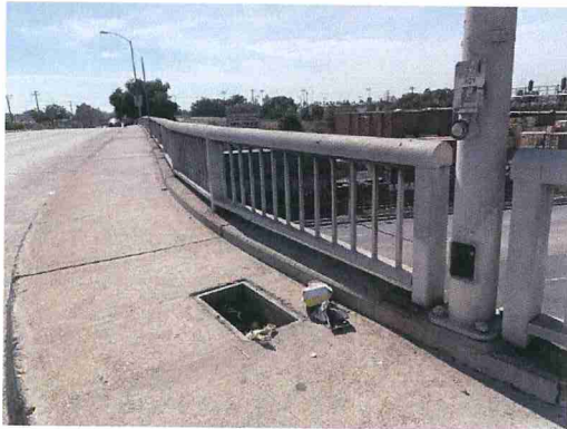
P4b_Missing utility boxes covers in light post and sidewalk (pic from August)
