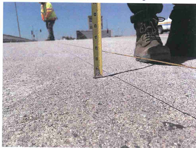
Photo 16 Buckling of Roadway
