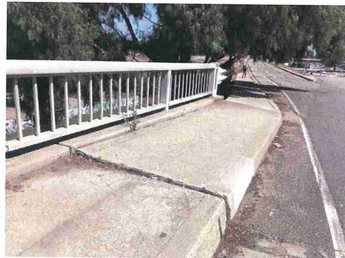
P5_Approach sidewalk settlement at N/E of bridge
