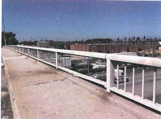
P3_Missing baluster in handrail _ Need repair
