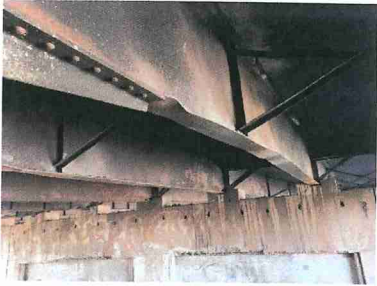
Girder 4- Lower flange and Bay 2 top bracing were distorted
