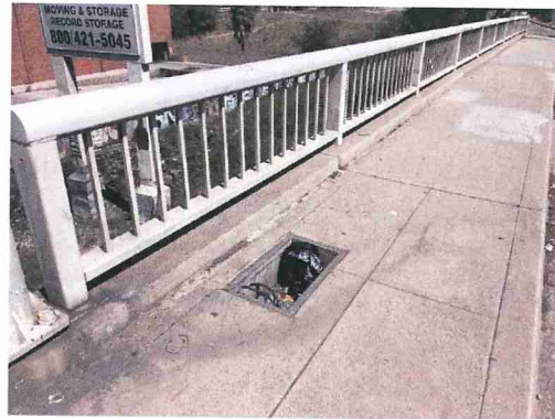
P4a_Missing utility box cover in sidewalk _ Need repair
