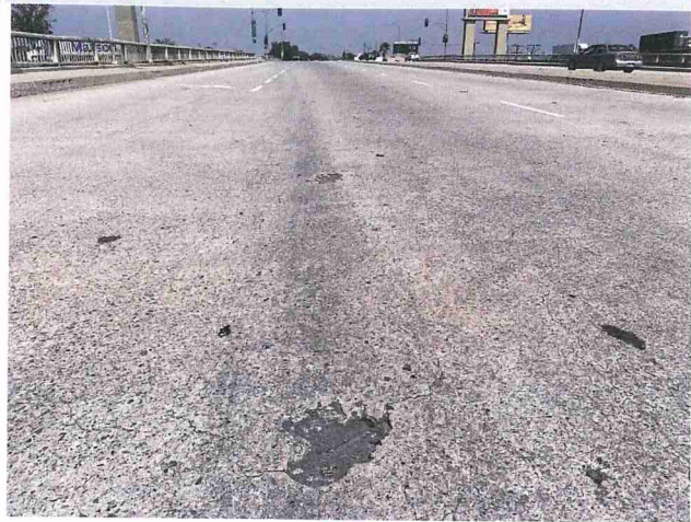
Photo 5 Deck Spalls and Cracking
