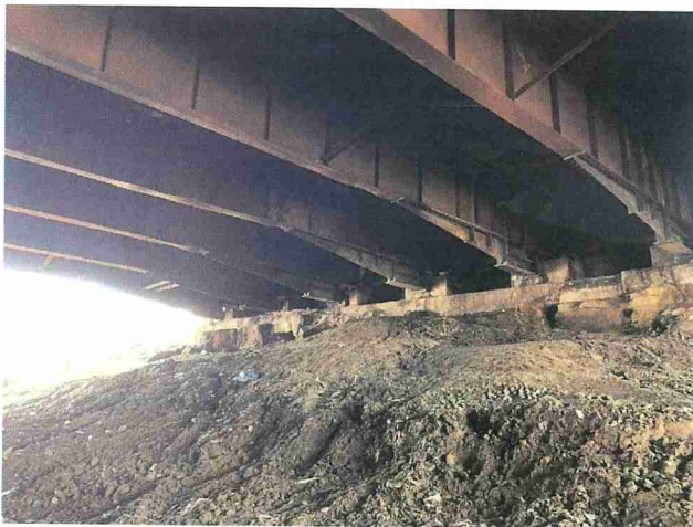
Photo 13 East Abutment Fire Site
