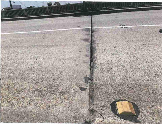
Photo 17 Burned Expansion Joint
