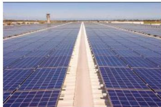
Figure 2: Rooftop View of Adelaide Airport Solar Installation
