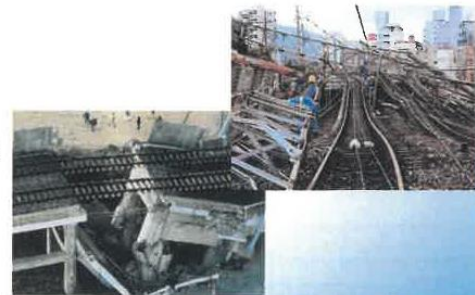
The great earthquake stroked in 1995. The urban railways were heavily damaged. But we rebuilt for only 74 days.
