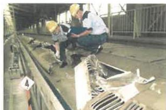
vehicle damage due to concrete peeling in the tunnel (1999)
