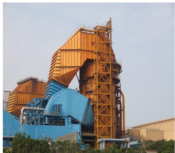
Desulfurization Equipment - Flue Outlet of Absorption Towers
