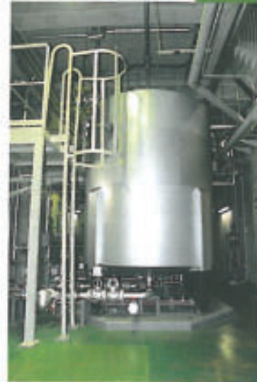
Drainage sterilizing tank
