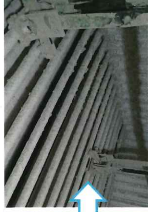
■ Cleaning with Shock pulse sootblower
