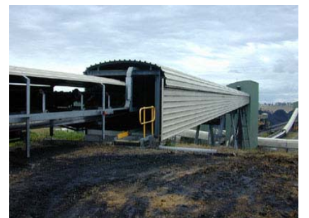
Entering crushing station
