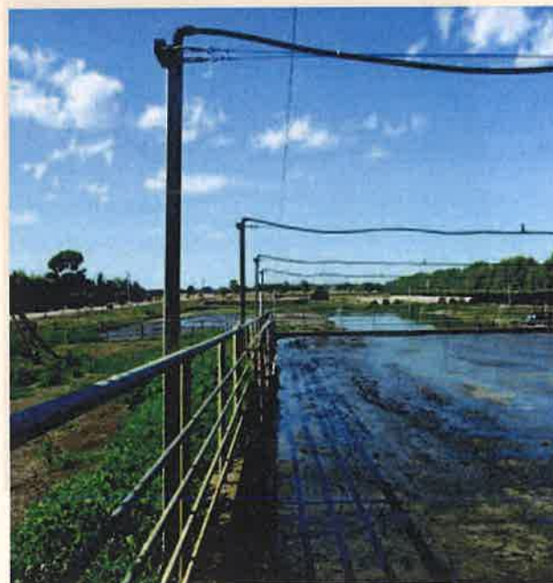
Steel posts that supports the water pipelines and allow the individual cables to be tensioned.
