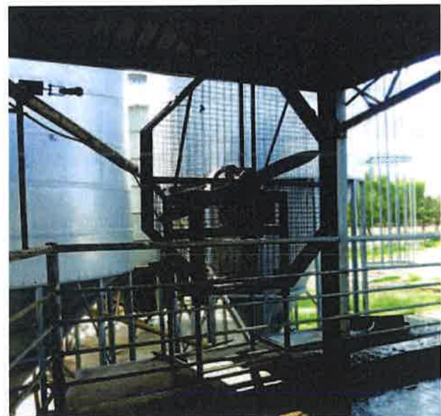
A large industrial fan can be used in conjunction with the spray curtain to keep air circulating in the dairy shed.
