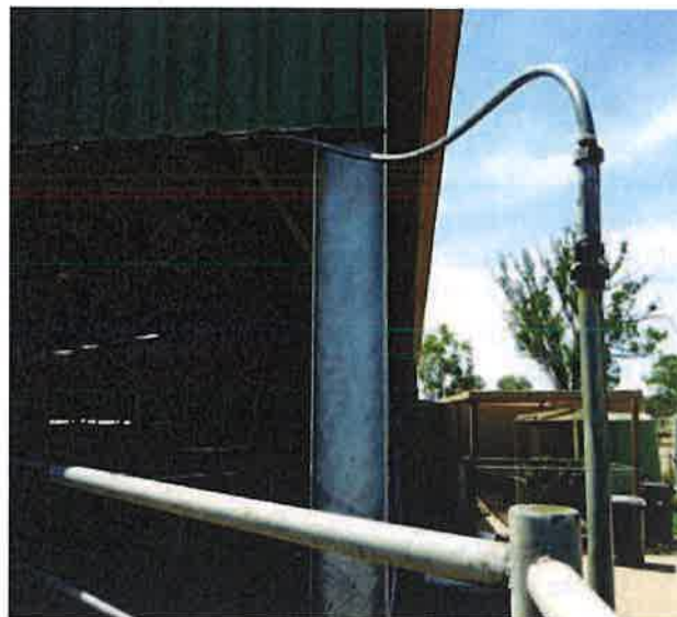
Spray curtain water supply and filter.
