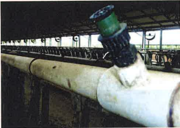
Sprinklers mounted above the head stanchions in a freestall barn. Droplet size can be adjusted.
