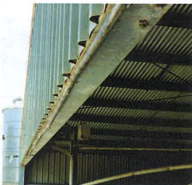
Polyethylene pipe attached to the dairy shed roof for the spray curtain.
