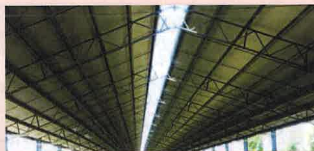
Pitched roof has a ridge vent to let heat and humidity escape. It also influences convective air movement.
