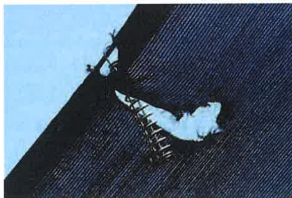
Damage to shade cloth caused by poor maintenance. Ensure that springs that become detached are re-attached as soon as possible.
