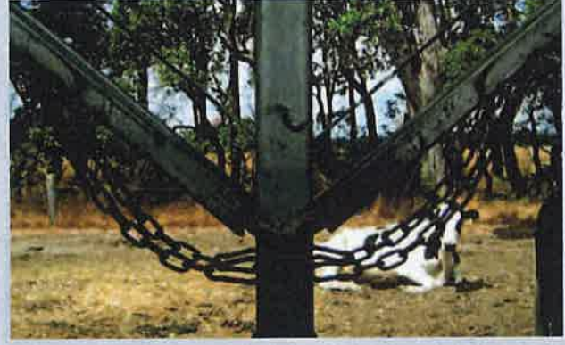
Chains used to prevent roof spans from being blown off the support trusses.
