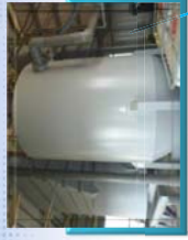
Sand Filter Tank
