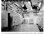
Control Room Control room for monitoring and testing DER systems.
