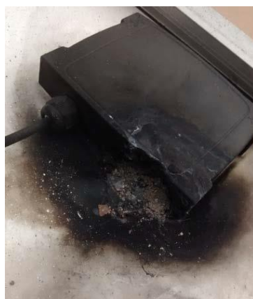
圖 9、PV module junction box showing scorching from internal arcing
