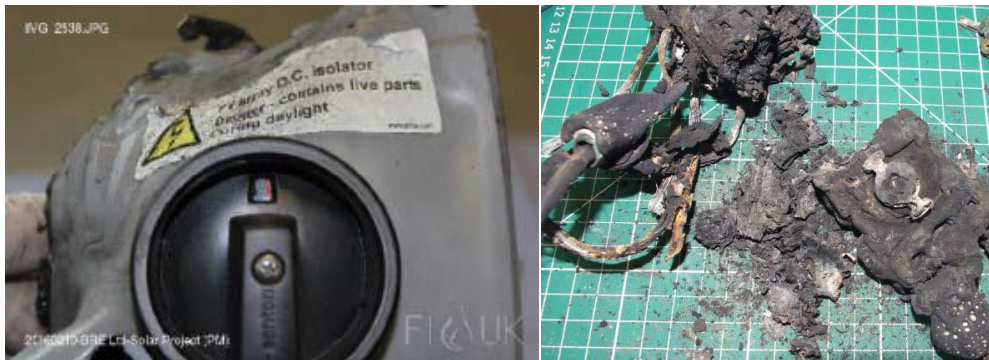
圖 7、DC isolators in different states of fire damage
