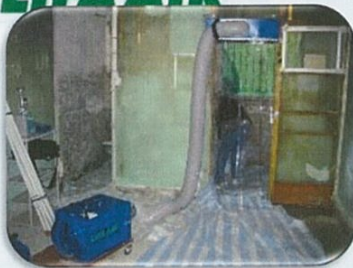
Cooperate with Housing Authority to sustain air quality to protect occupants and workers during repair and renovation
