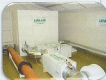
Air filter testing lab
