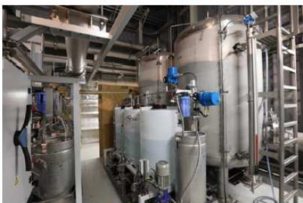
Valve Cooling plant
