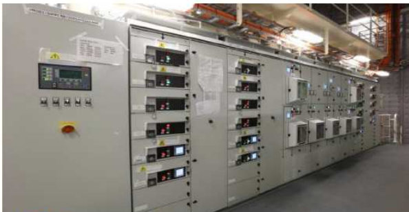
Emergency Distribution board
