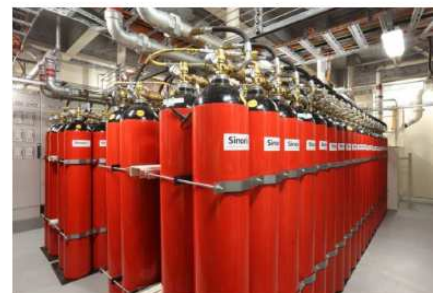
Fire Fighting gas plant
