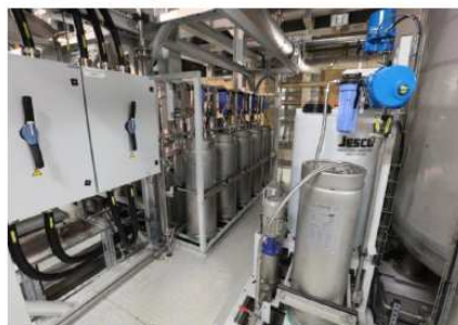
Valve Cooling plant
