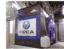
Advanced Cogeneration Engine
