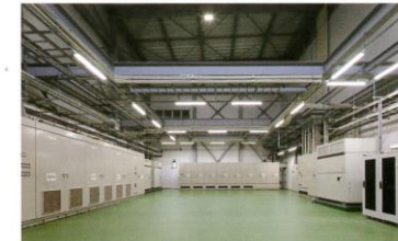
Grid Connection Testing Facility
