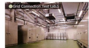
Grid Connection Test Lab.S This laboratory is available for grid connection tests within a range from small and multiple medium-size inverters to a large-size inverter of 1.5MW.
