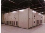
Grid (AC) Simulator AC power source (up to 5000 kVA) with 400V and 6000 bus to connect and test DERs including anti-islanding test and Fault Ride Through (FRT) tests.
