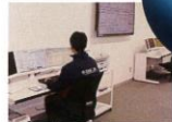
Central Control System (2F) It manages and monitors all power equipment to ensure safe operation.
