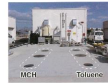
Large storage tanks
