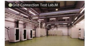
Grid Connection Test Lab.M The largest grid connection test laboratory in Japan accommodating a 20-foot-long container to conduct grid connection tests for up to 1.5MW, and simulation power distribution line.
