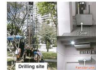
Ground-source heat pump (GSHP) system installed at Chulalongkorn University, Thailand
