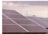
Solar Photovoltaic Array This facility has the capability to connect an outdoor 250kW PV system to compare the difference between a PV array simulator and a real PV array system.
