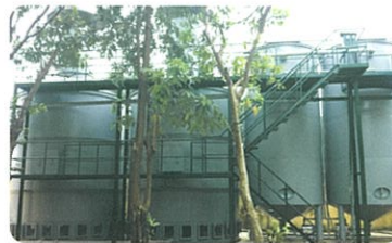
Wastewater treatment plant in Hanoi Milk JointJoint Stock Company
