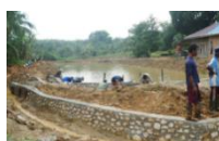
Water Reservoir 686 Unit
