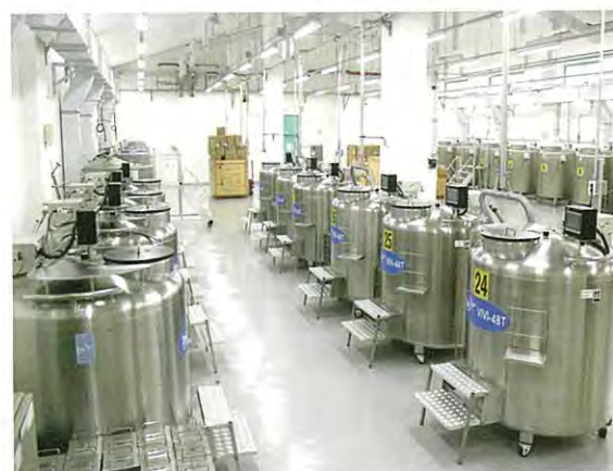
Cryogenic liquid nitrogen freezers
