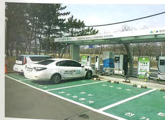
Electric vehicle charging station
