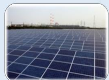
Photovoltaic Power Plant
