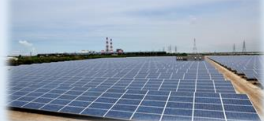
Yongan PV Project ( 4,637kW ) by Fortune Electric
