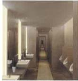
圖19 在洗手間中裝設節水的衛生設備 Figure 19 Use of water saving sanitary fittings in the toilet
