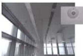
圖17 在辦公室中安裝廣度感應器 Figure 17 Application of photo sensor in office
