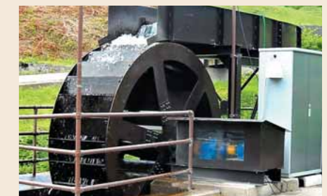
Small hydroelectric power generation
