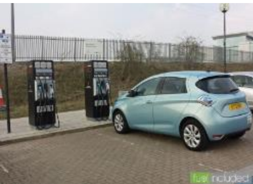
City-wide network of 50 rapid chargers 整个城市网络的50个快速充电器
