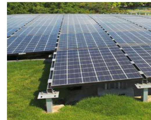
Virtual power plant, Munich
