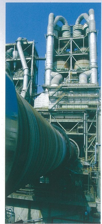
Suspension pre-heater and rotary kiln
