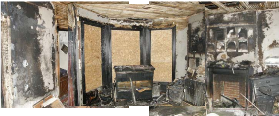
Front Room (Room where firefighters were burned)
