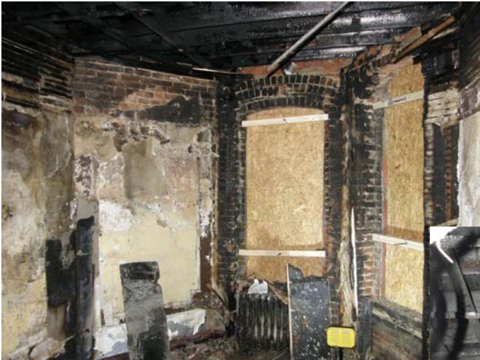
Rear Room (Room of fire origin)
