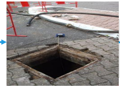
Check the LEL on the pit
