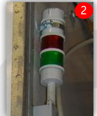
Light & Audio ground safety signals
