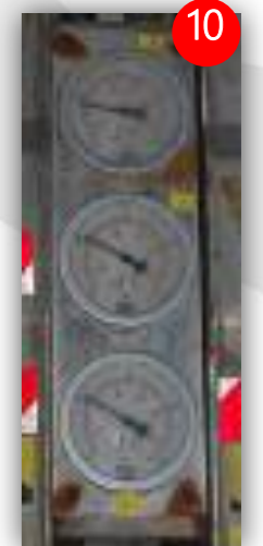
Manometers of the 3 tanks
