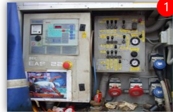
Electric & pneumatic board
