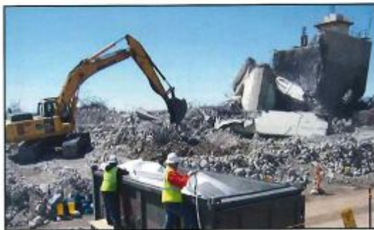
Workers close-up a container of low-level radioactive waste debris from the demolition of the Reactor Maintenance, Assembly, and Disassembly Facility used for nuclear rocket development at the NNSS in the 1960s.
