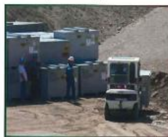
Workers place a metal box containing mixed low-level radioactive waste in a disposal cell at the Area 5 Radioactive Waste Management Complex located in the southeast portion of the NNSS.
