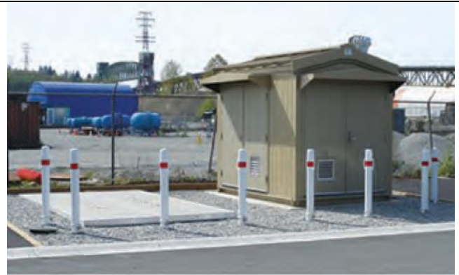
A 23 kW PRV Hydro project, recently constructed in the District of North Vancouver.
