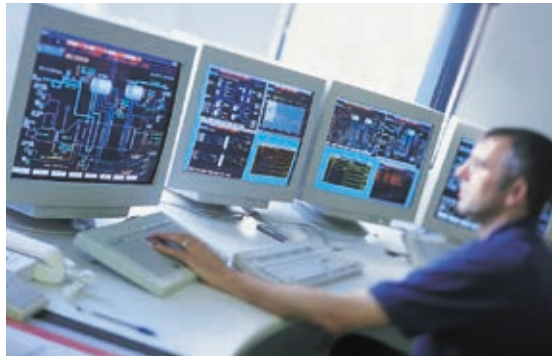
All processes at the power plant are monitored via the central control room
