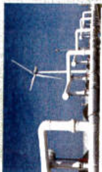
FUKASHIBA Sewage Treatment Plant
