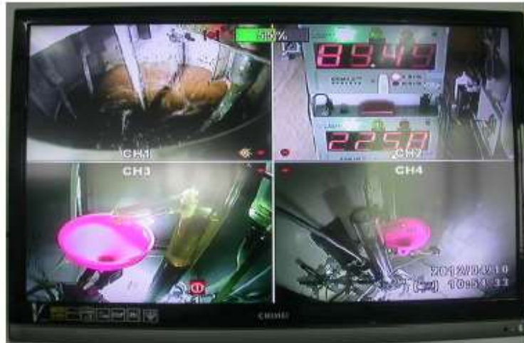
Fig. 4. Monitoring system of waste solution treatment facilities
