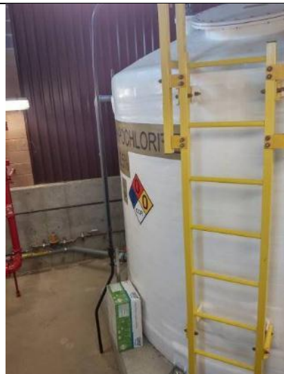
Foothill 淨水場次氯酸鈉藥槽
