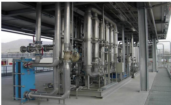
The Ultrafiltration system is equipped with SS-TiO 2 Tubular membranes treated water is suitable for Reuse, eg. Agriculture
