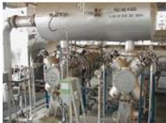
Kobelco / Refining / Residue desulfurization (RDS)
