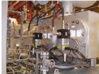
Dresser Rand / Refining / Hydrodesulfurization (HDS)
