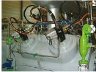
Neuman & Esser / Chemical / Chlorine electrolysis
