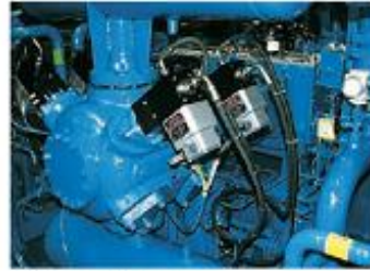
Ariel / Gas turbine plant
