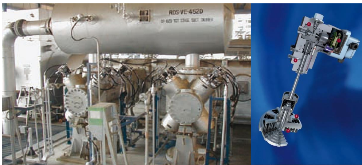
Kobelco / Refining / Residue desulfurization (RDS)
