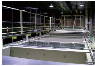
Chemical decontamination operating line
