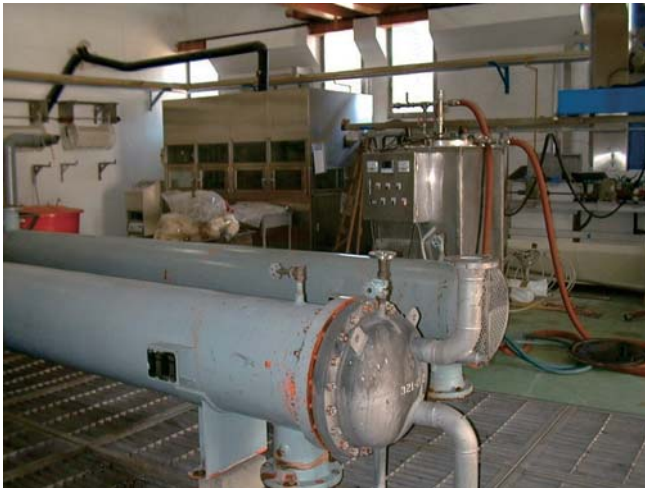
Clean heat exchange with a circulation system
