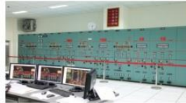
Shian Duh E/S Control Room
