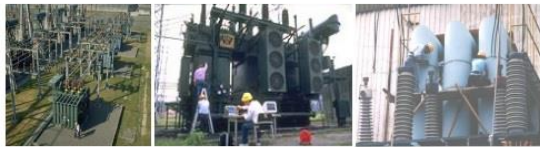
Transformer, G.I.S., ...etc.
