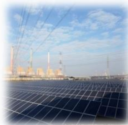
Taichung Longjing PV Project ( 6,486kW ) by Allis Electric, etc.
