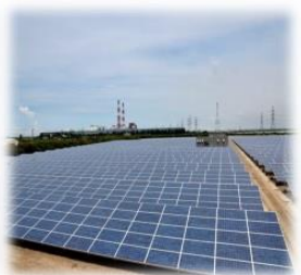
Yongan PV Project ( 4,637kW ) by Fortune Electric
