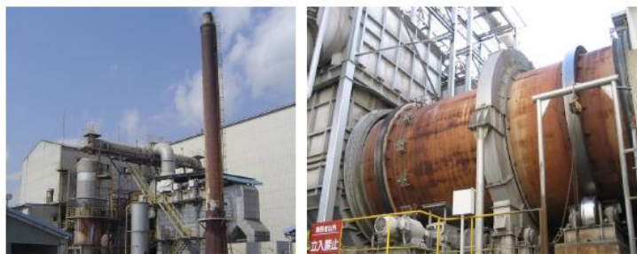
Example of Treatment Facility
