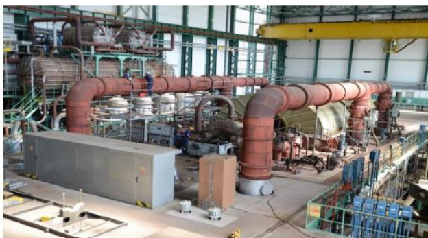
TG 22 before dismantling
