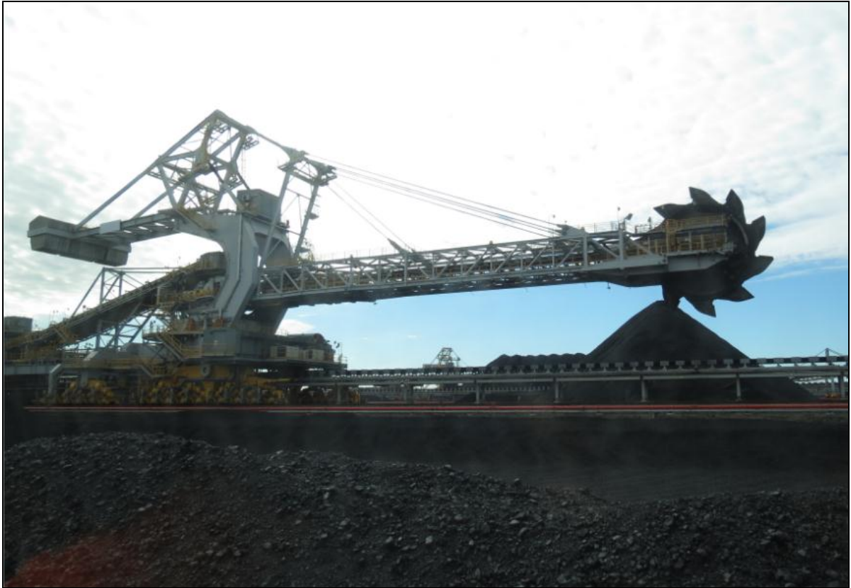
圖168 NCIG 斗輪式堆/取煤機(Bucket Wheel Stacker/Reclaimer)
