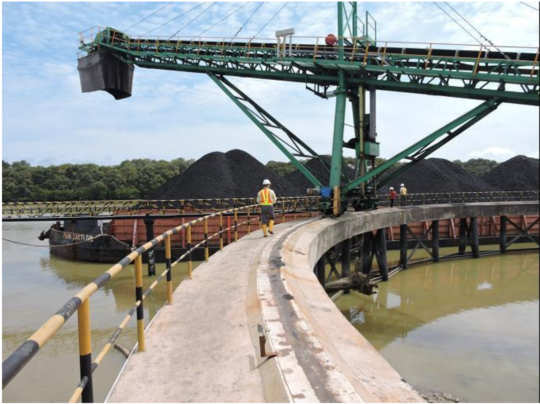
圖88 Lebanon Jetty Radial Conveyor
