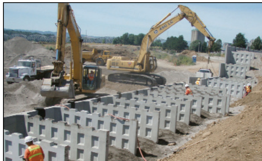
Two excavators working at the same time - one setting and one backfilling
