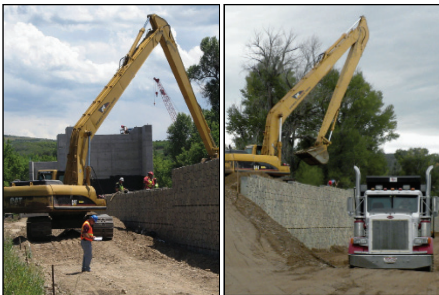
Long boom excavator – working in front of the wall and working on top of the back-to-back walls
