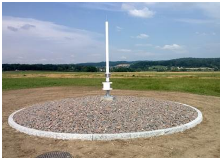
Reference GBAS antenna in Zurich, Switzerland
