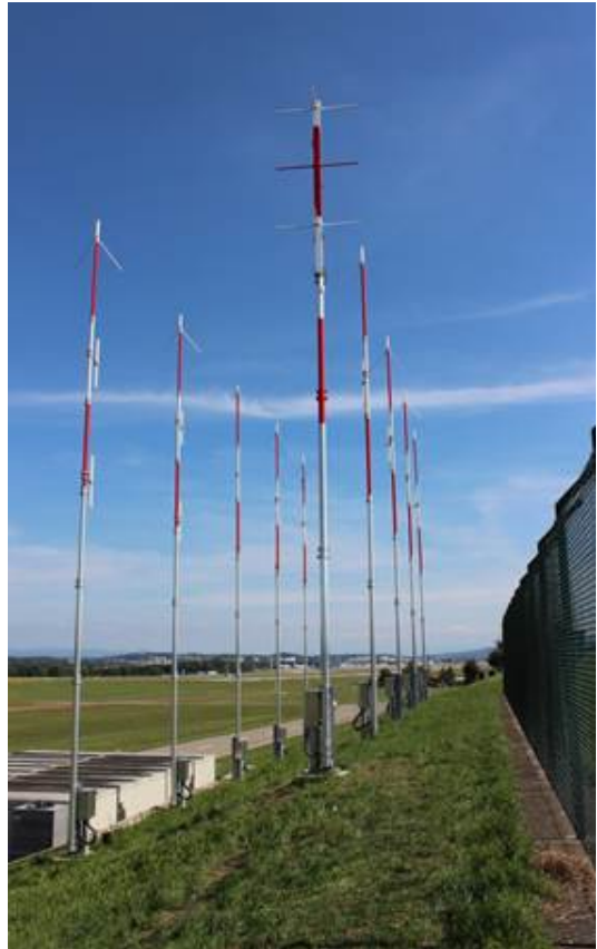
VHF antennas of the Zurich GBAS
