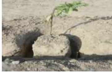
Installation of circular lateral pipe along with emitters around the guava tree
