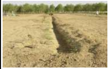
Installation of lateral pipe along with the emitters around the guava tree for utilization of sewage water through drip irrigation
