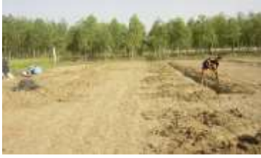
Installation of lateral pipe of subsurface drip irrigation system to utilize sewage water
