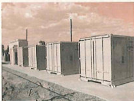
Fig.11: 0.8MW-class Lead Acid Battery system in container
