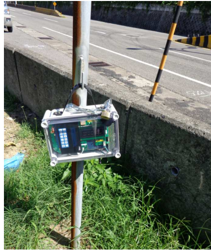
Mobile radiation monitor box is hanged on the hook of the pole
