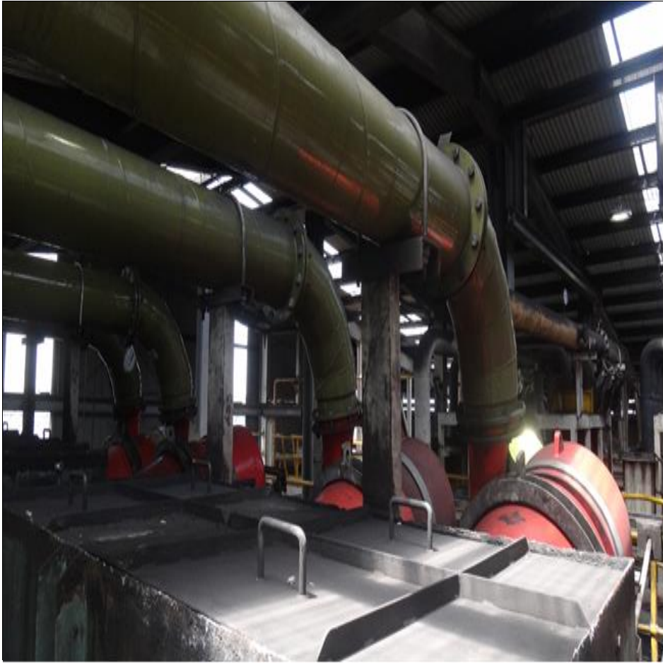
Clarence 礦區洗 煤廠去水設備 (dewatering equipment)
