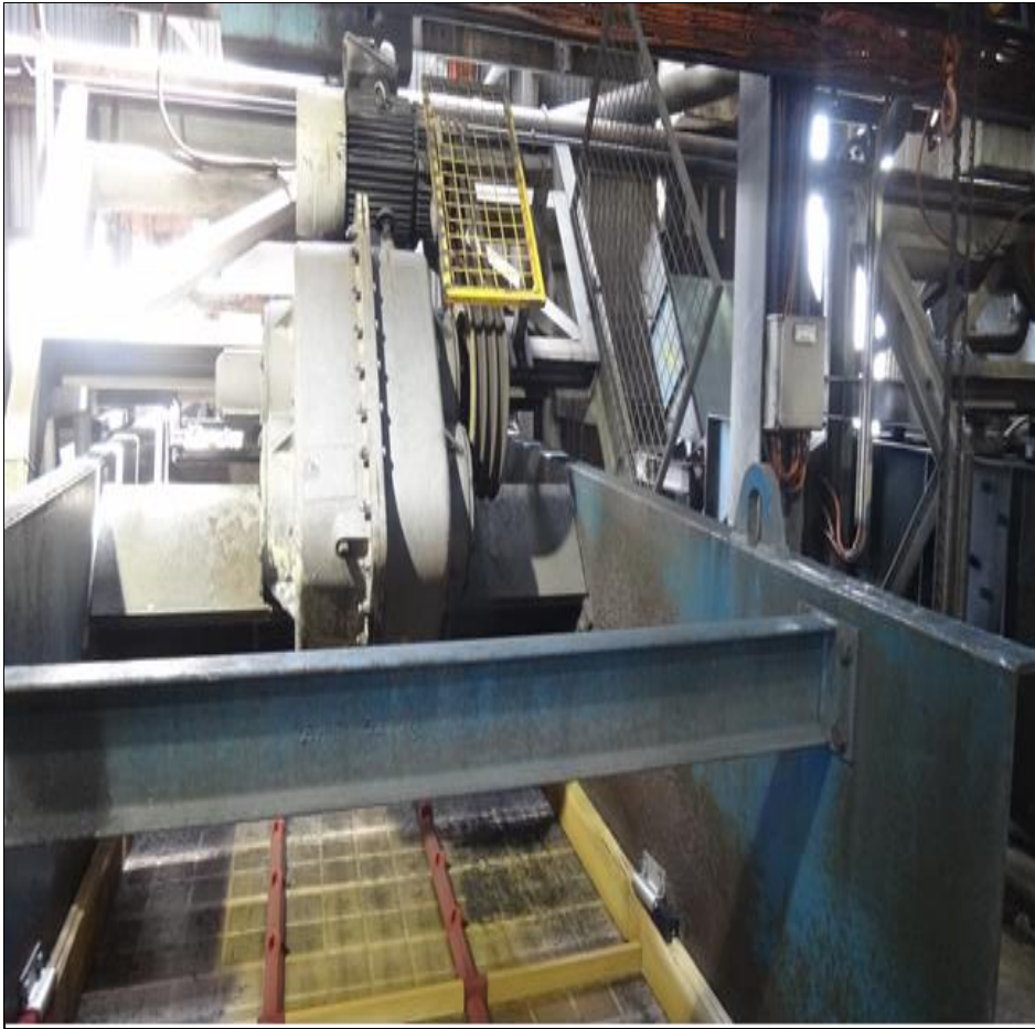
Clarence 礦區洗 煤廠過篩設備 (screening equipment)
